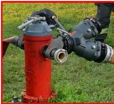
Hydrants are maintained regularly
