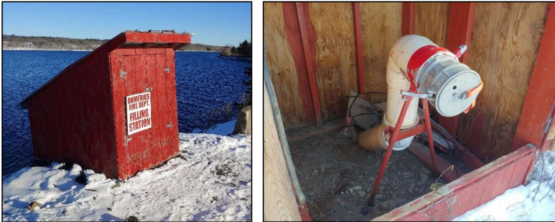
Figure 2: Dry hydrant filling station in Dumfries along route 102 that feeds from the Wolastoq - Saint John River.
